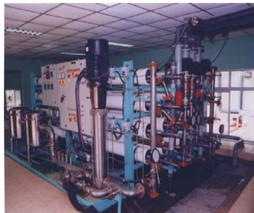
1 MLD Indigenous RO Plant at CPCL, Chennai
