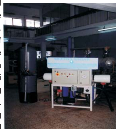
Picture of 1000 LPH brackish water RO plant installed in Ervadi village, Ramanathapuram District in May 2004
