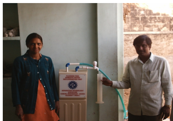
Defluoridation unit at Bhatvas, Mehsana District, Gujarat
