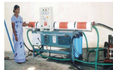
2000 LPH RO plant installed at Akkarapattai village of Nagapattinam District, Tamil Nadu.
