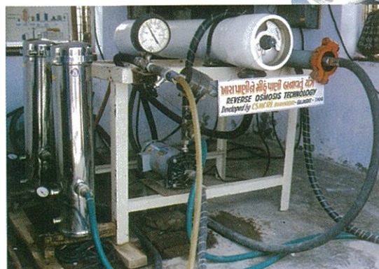
RO plant installed at Kalyanpur village for field testing of indigenous 200 mm (8½) TFC module.
